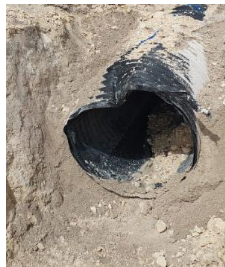
Datalnama area - Damaged pipe
