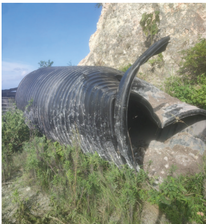
Lamlangil area - Damaged pipe
